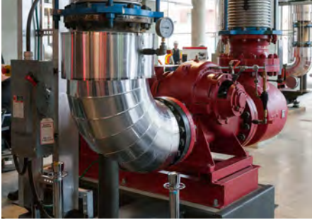
District energy plant in East Village
