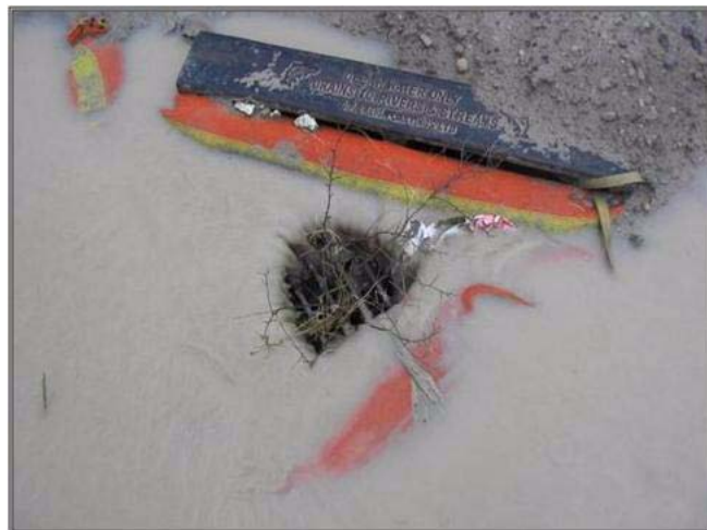
Figure 9-5: Failed Storm Inlet Protection
