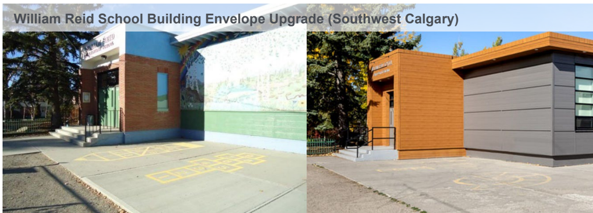
Figure 1.0 – The William Reid School removed the entire building exterior and replaced it with a high performing building envelope. Photo courtesy of ACE
