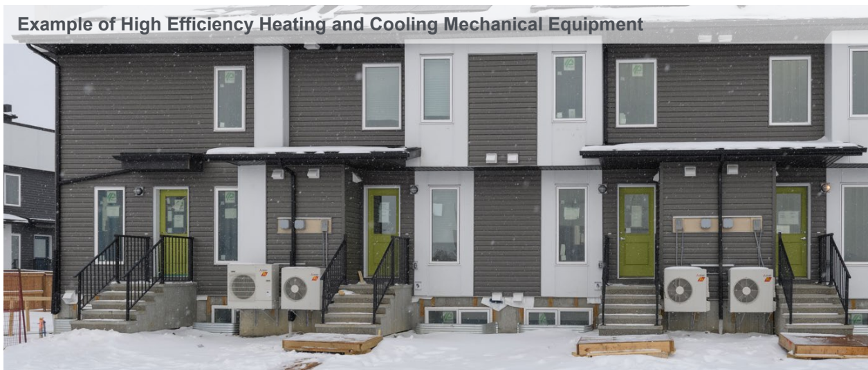
Figure 3.0 – Electric heat and cooling pumps are energy efficient mechanical solutions. However, unlike a more conventional gas-powered furnaces, electric heat pumps require access to fresh air and therefore need to be located outside. Photo courtesy of City Manager's Office
