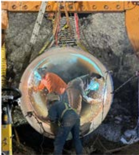
Aging, critical infrastructure
