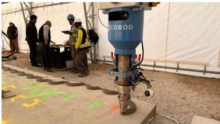
The Siksika Nation is using a large 3D printer, which includes a 4-foot tall robotic arm, to build a group of fourplexes that will be used as transitional housing. (Radja Mahamba/CBC News)
