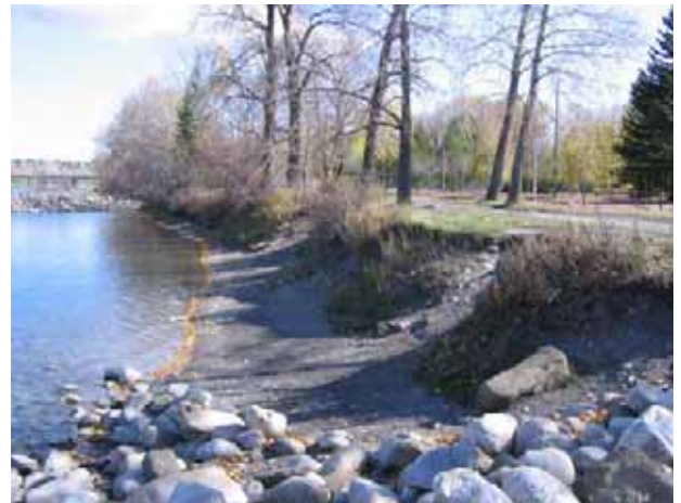
Eroded bank between groynes.
