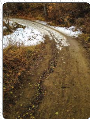
EROSION CAUSES AN UNEVEN TRAIL SURFACE
