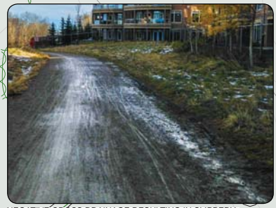
NEGATIVE CROSS DRAINAGE RESULTING IN SLIPPERY CONDITIONS AND EROSION AND POTENTIAL FOR WINTER ICING
