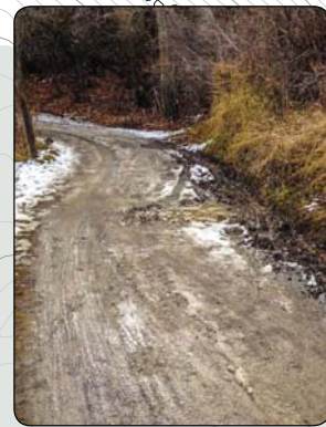
NEGATIVE CROSS DRAINAGE RESULTING IN SLIPPERY CONDITIONS AND EROSION AND POTENTIAL FOR WINTER ICING
