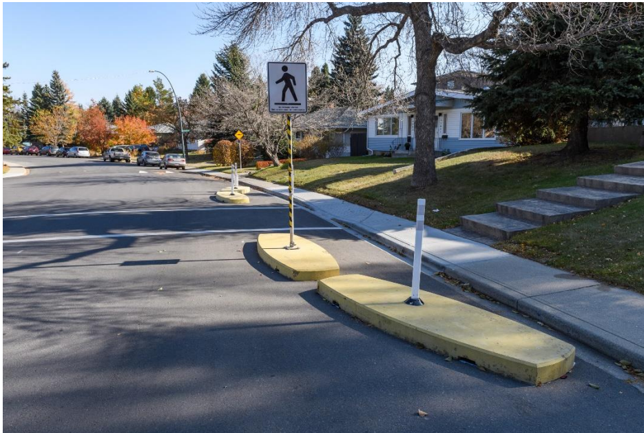
Figure 2. Temporary traffic calming curbs at Rosehill Drive and Rosewood Road
