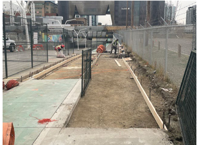
Looking north at the Remington access construction work, north of Olympic Way S.E., and 11 Avenue S.E. intersection
