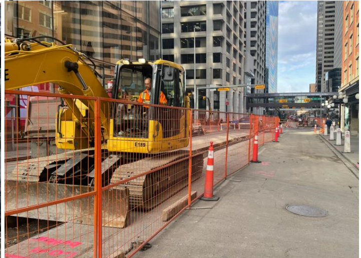
Looking North at Enmax duct bank installation along 1 Street SW, North of 7 Ave SW
