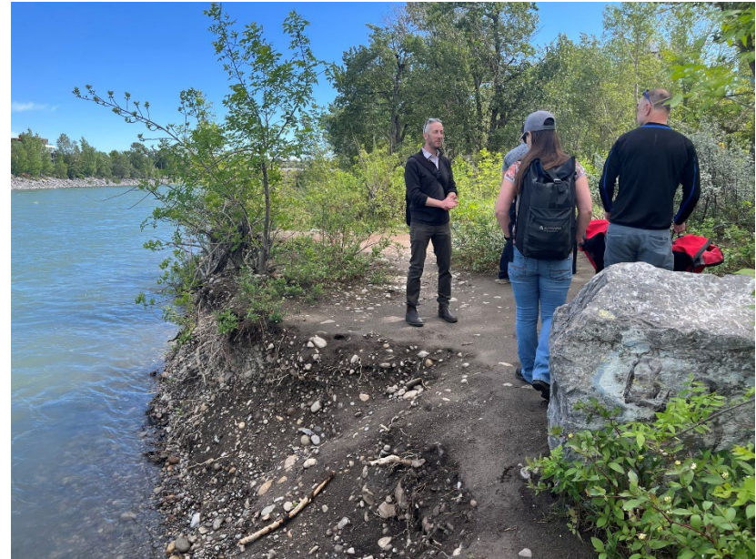
Photo 2. Eroded and compacted riverbank on the south bank east of 10 Street.
