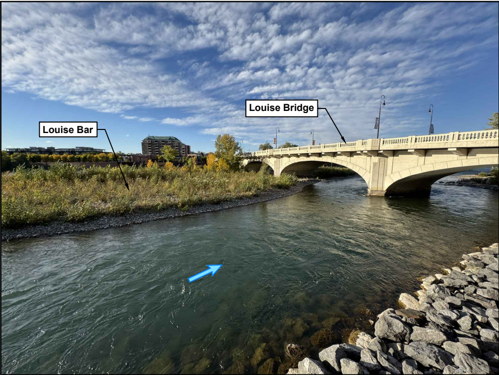
Photo 15: Louise Bar is obstructing two of the bridge spans. September 18, 2024.
