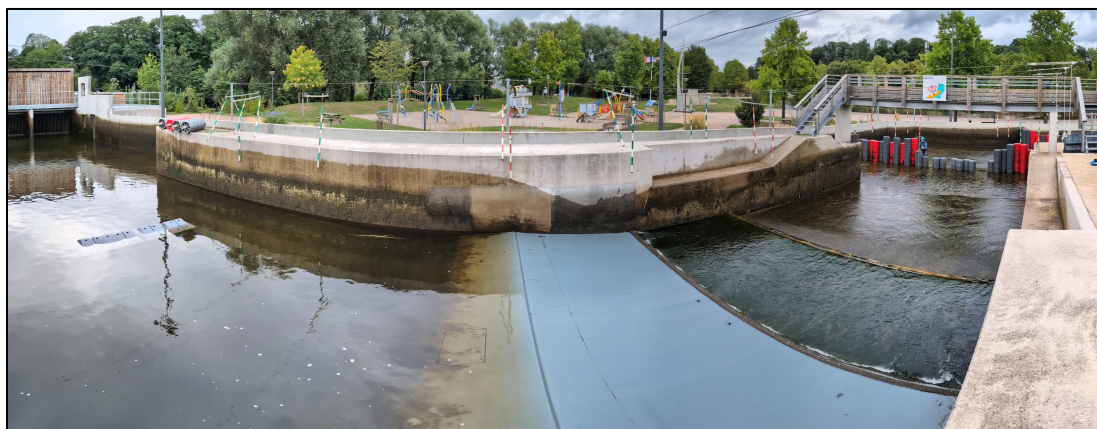
Figure 24: Epinal, France, flap gate with downslope lowered.
