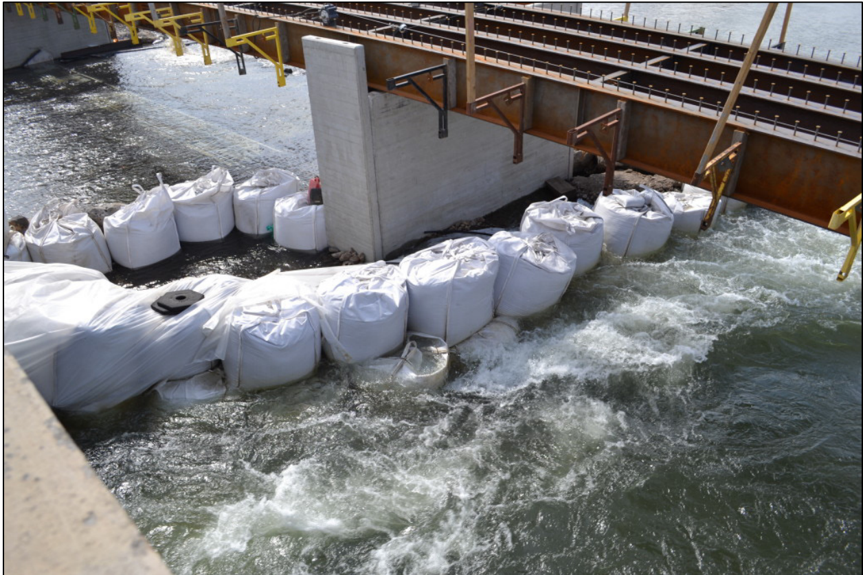
Figure 57: Meter bags at the Bend Whitewater Park, USA.
