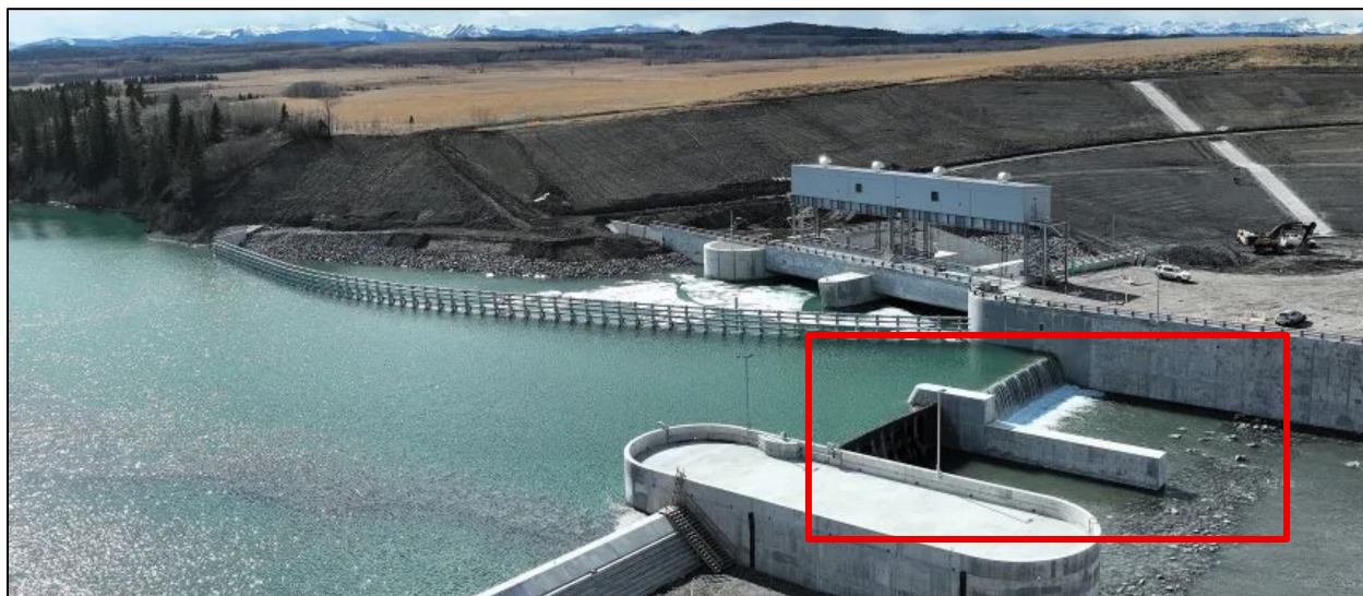
Figure 13: 5m high pneumatic flap gates as part of the Springbank Off Stream Reservoir. 7
