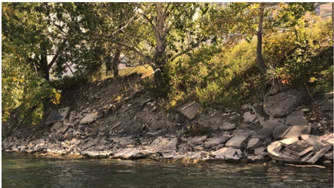
Figure 9: Existing riverbank along the south slopes, with concrete debris and active erosion
