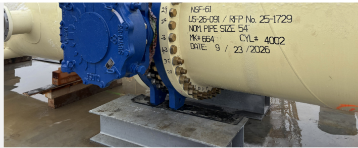
New valve and pipes ready to be installed at the Shaganappi Pump Station.
