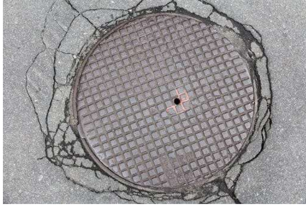
Figure 3.5: Cracked Surface Surrounding a Manhole 4
