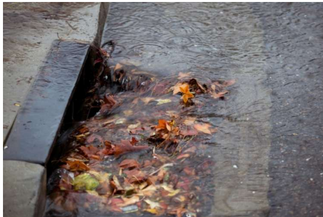
Figure 3.6: Catchbasin Intake Restricted by Leaves 5
