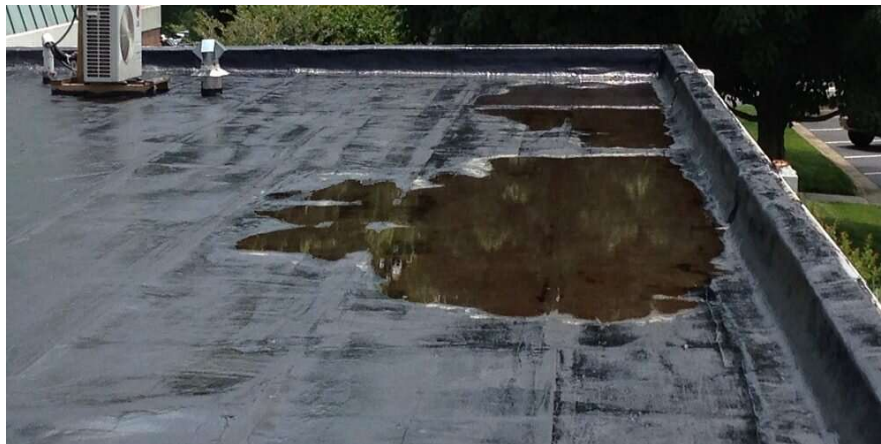
Figure 3.13 Ponding on Roof 11
