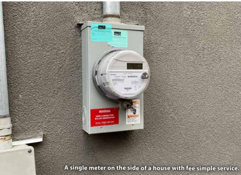
A gang meter base on the side of a townhouse.
