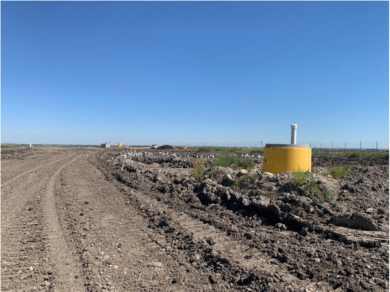
Figure 38. Example of a Landfill Leachate System Access Riser Assessed During the Field Investigation
