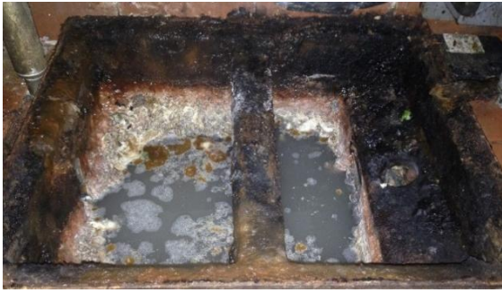
Figure 8 – Example of a grease interceptor that has not been properly maintained. The visible corrosion suggests the interceptor no longer functions properly.
