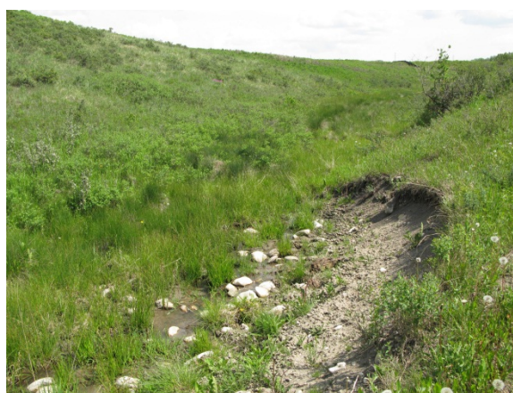
Photo 5 – Localized erosion of the west bank of Coach Creek in the NW¼ 31-24-2-5.
