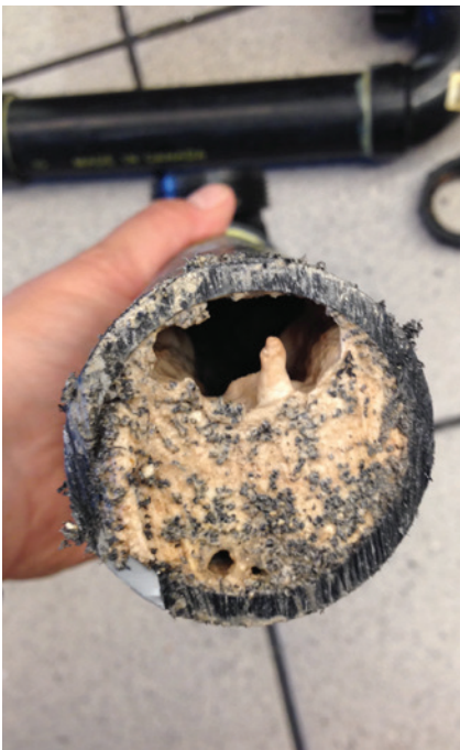
Pipe almost completely blocked with FOG
